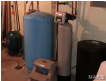
Back flush water filter, pressure tank, water softner
